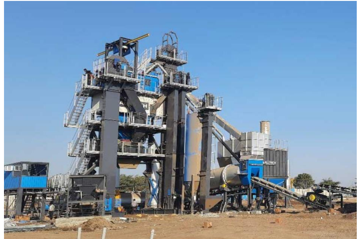
Asphalt mixing plant
